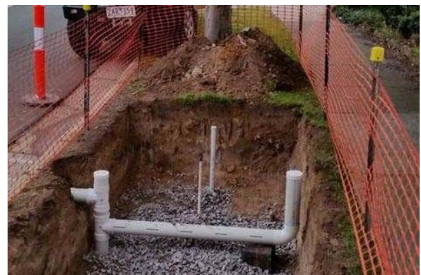
Figure 1. An infiltration trench being retrofitted alongside an established tree. The pipework conveys water from the kerbside into the trench which will be filled with gravel. The trench can hold ~1500 L of stormwater - supply the tree with enough water to maintain transpiration during summer and reducing stormwater runoff by ~50%.
