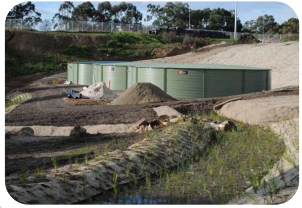
Above: construction of rainwater tanks and rain-gardens nears completion at Morrison Reserve.
